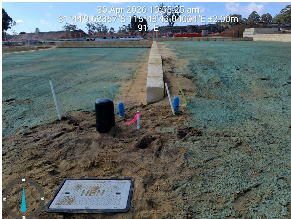
Plate 6: Reticulated water has been installed at the time of assessment.
