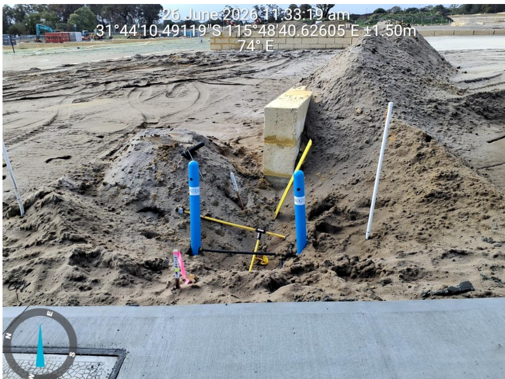
Plate 6: Reticulated water had been installed at the time of assessment.
